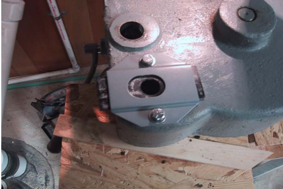
Figure 8 – retainer assembled to gearbox (note that the retainer is erroneously upside-down in this photo – the shaft hole should be toward the bottom of the gearbox)
